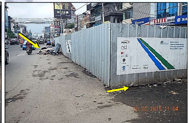
Blok A Station : Waste Cleaning Required
