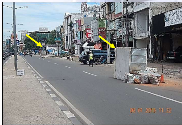
Haji Nawi Station : Reinstatement of Utility Excavation Required
