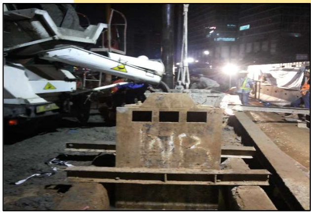
Setiabudi Station : D-wall panel no P30 under pouring concrete at east side
